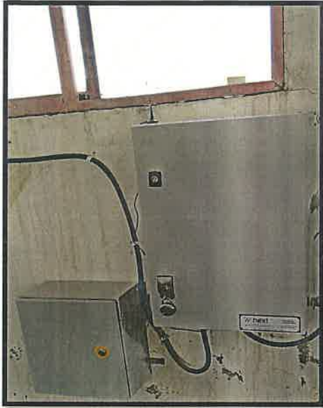
Location:- DRAINAGE PUMPING PS-1
