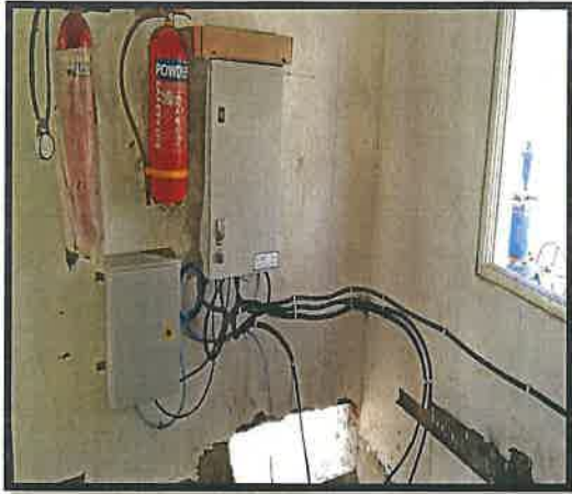
Location:- Pumping Station A1
